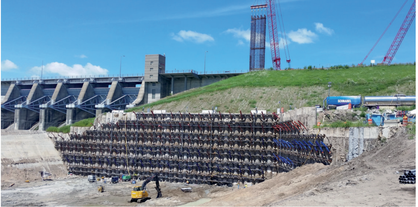
Secant pile wall for powerhouse construction (at front), with diaphragm wall cage being lifted for upstream placement (background)
